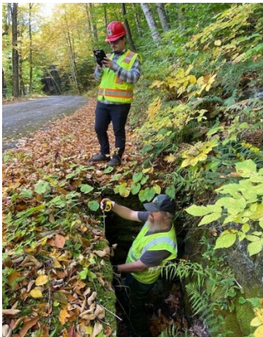
USDA Forest Service Photo 3 Archaeological Technician, Brandon Emerson (Left) and Engineering Technician, Seth Coffey (Right) conducting measurements of the Civilian Conservation Corps-era culverts on Forest Road 10, Mt. Tabor.
