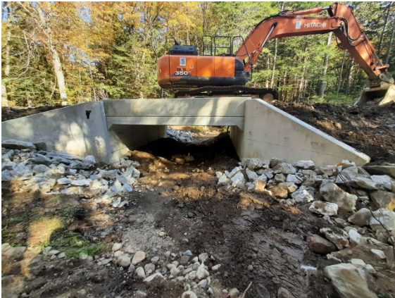
USDA Forest Service Photo 5 Construction of an aquatic organism passage culvert replacement on Forest Road 10. USDA Forest Service photo.
