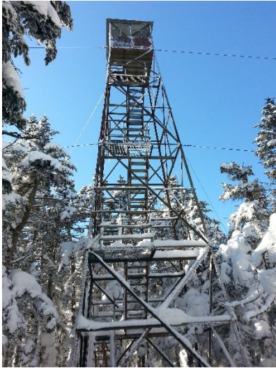
USDA Forest Service Photo 6 Glastenbury Observation Tower remains closed to public use due to safety concerns.
